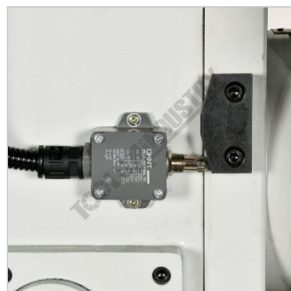
Mill Head Limiter Safety Switch
